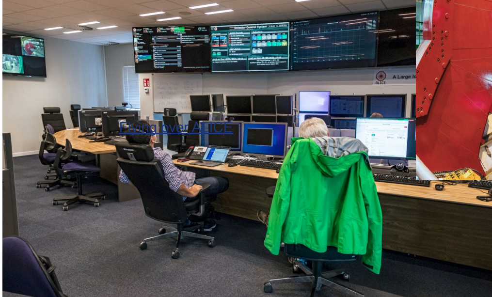
ALICE control room
